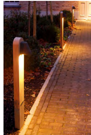
Fig. 37: Low level bollard lighting
