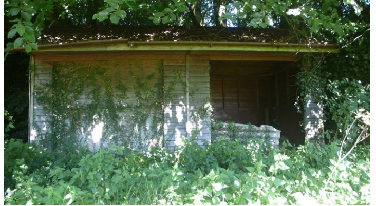
Photo 14: view showing the timber storage shed building in the north-western corner of the site.
